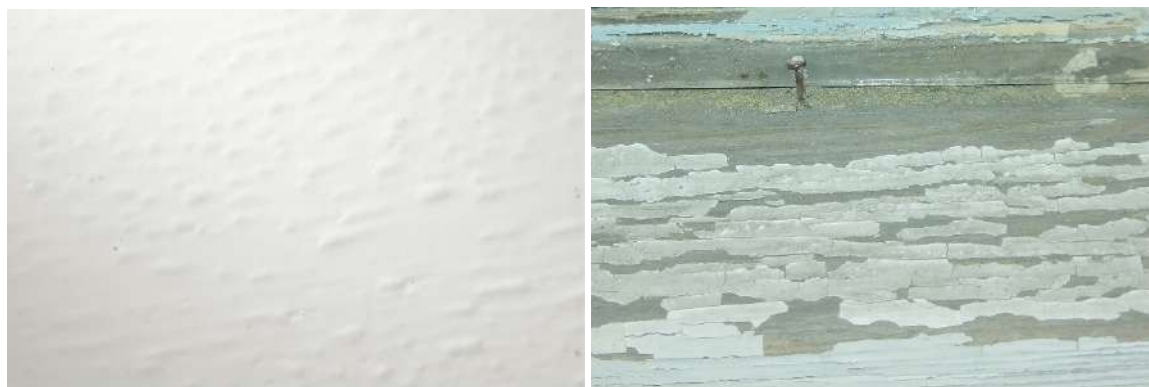
Figure 4: Failure in adhesion: a) water bubbles; b) flaking of the coating (Palija, 2020)
