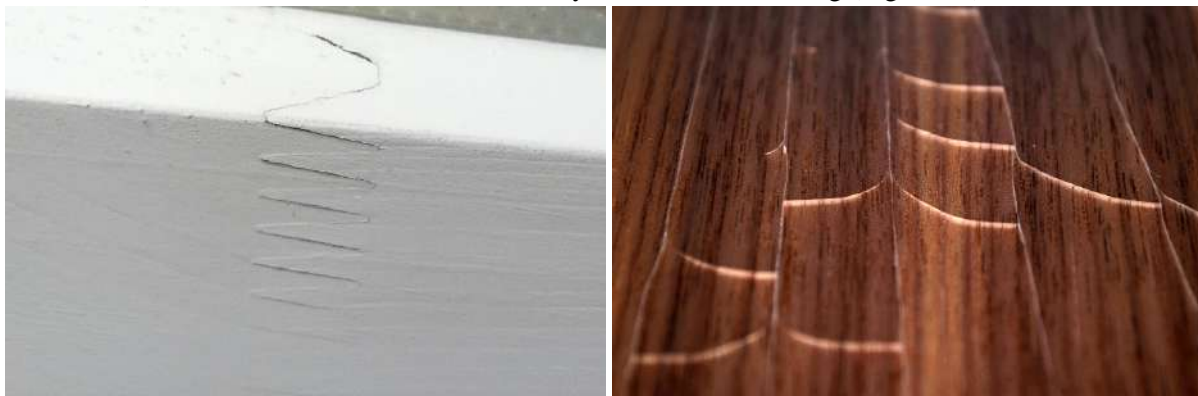
Figure 3: Cracks: a) along finger joint on the window frame; b) caused by low elasticity of the coating film (Palija, 2020)
